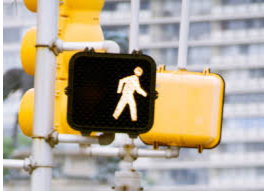
Figure 20. Example Pedestrian Crossing Signal.
